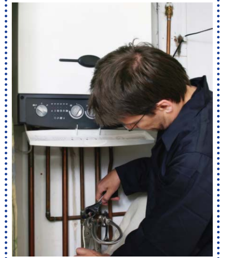
Above: Gas inspections keep you and your family safe.
